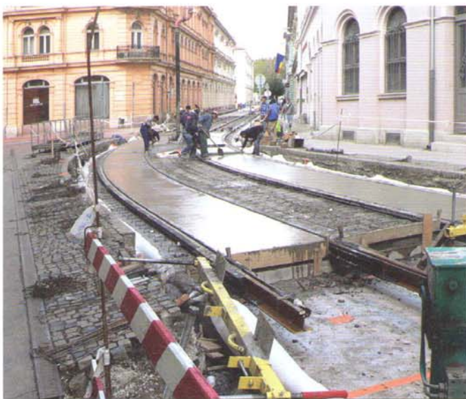
Szeged, city centre, line I; EPC vibration damping fibre-reinforced concrete, structural and track disk cover. CDM system superstructure
